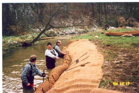
Installing fiber mat to help stabilize Rocky Run stream bank. See the special photo feature at the bottom of this webpage.
